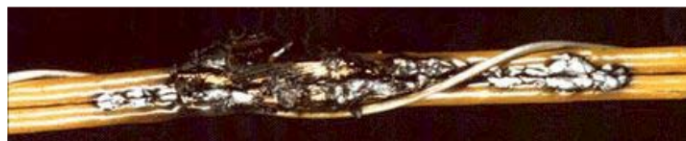
Figure 30: Example of arc tracking
